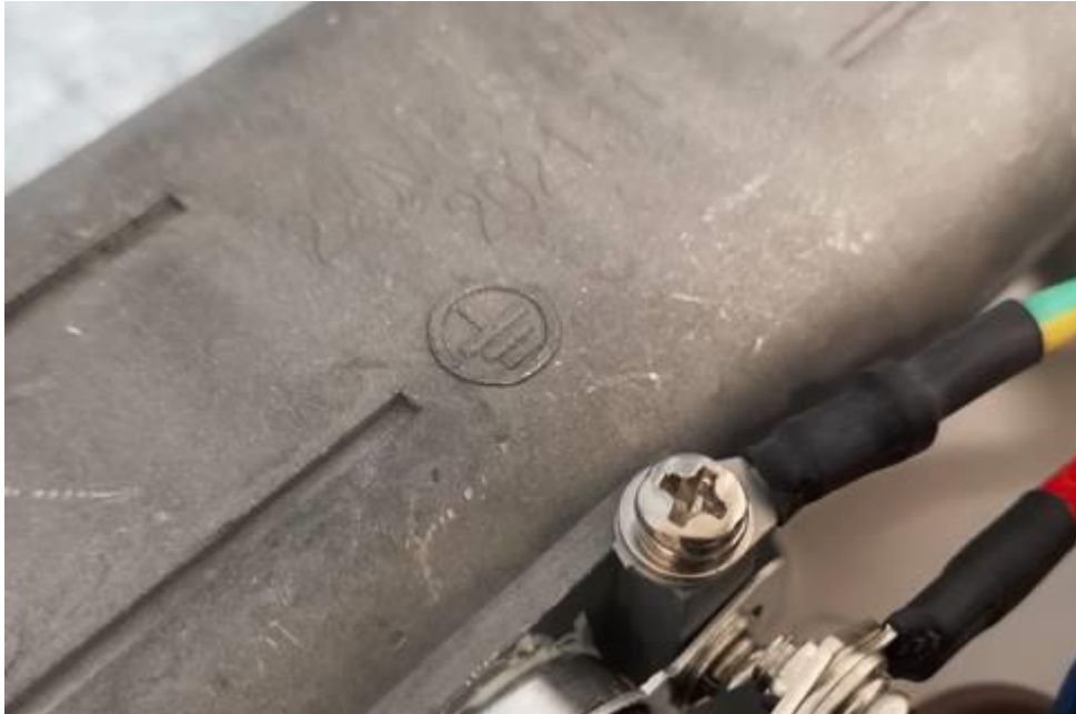
Earthing terminal view
